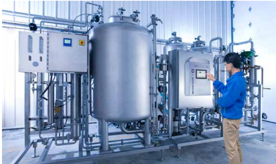
Field service engineer is commissioning the 7000RMS installed on the water system skid.
